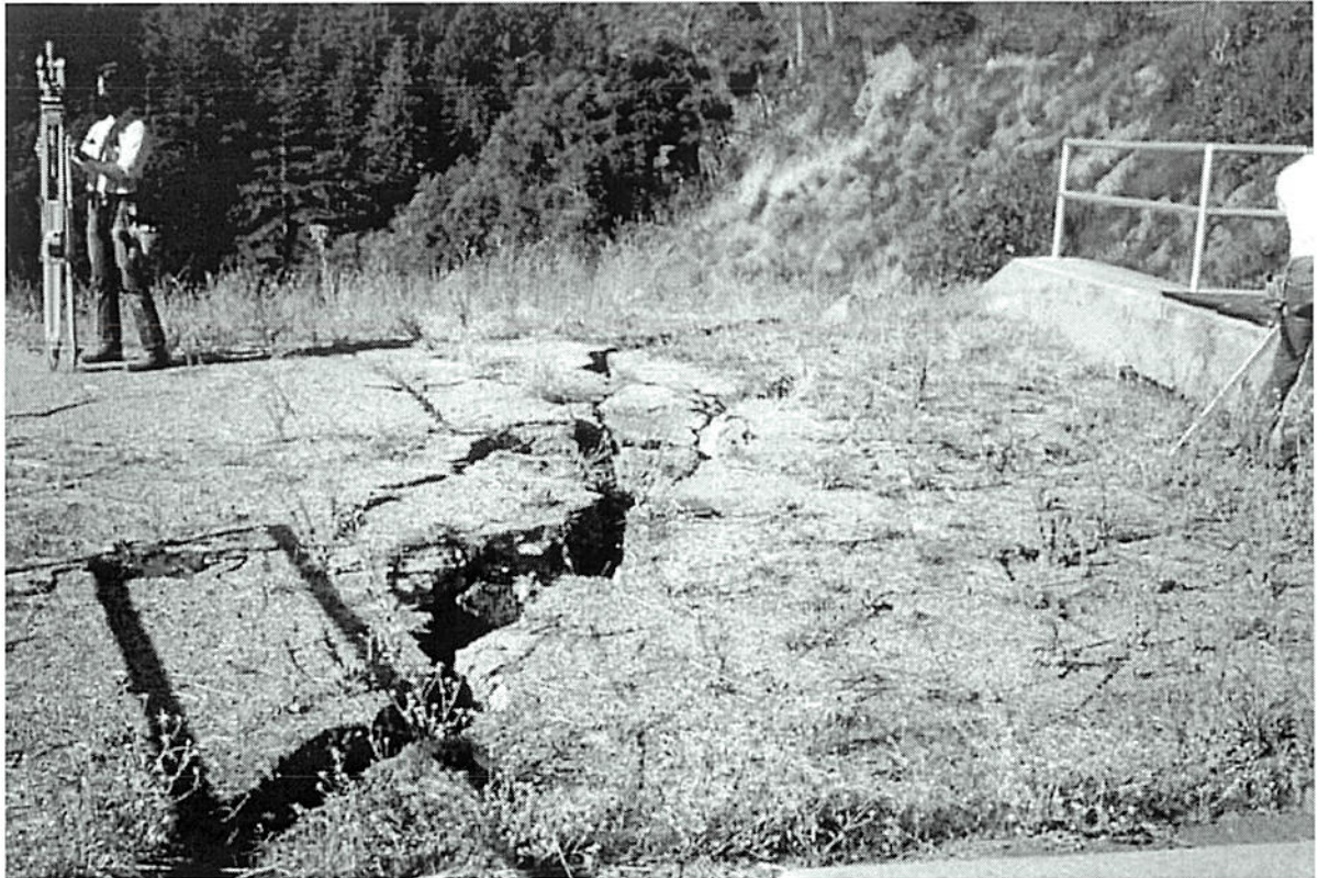
Figure 24 Photograph of transverse cracking adjacent to the spillway chute at Austrian Dam (U.S.G.S)
