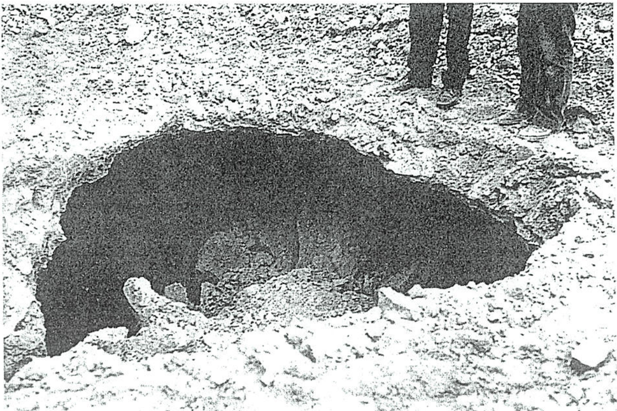
Figure 7 - Right Abutment incident during first filling
