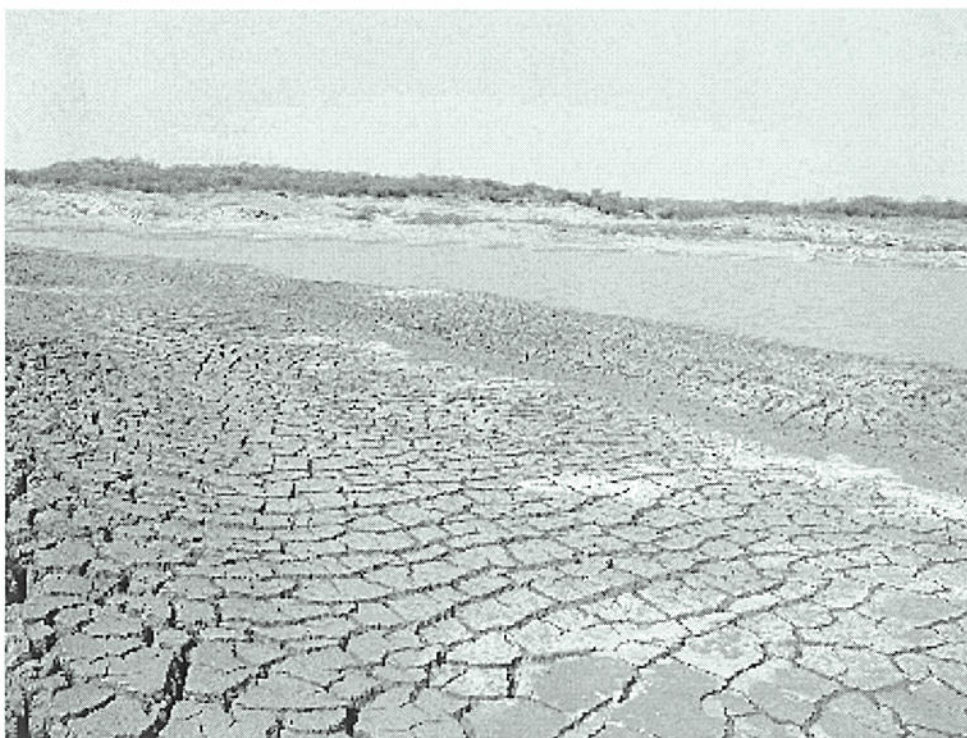
A bulge occurred at the upstream toe. A local farmer just upstream of the dam reported that water issued from ground fissures for approximately 0.5 hours on the day of the earthquake.
