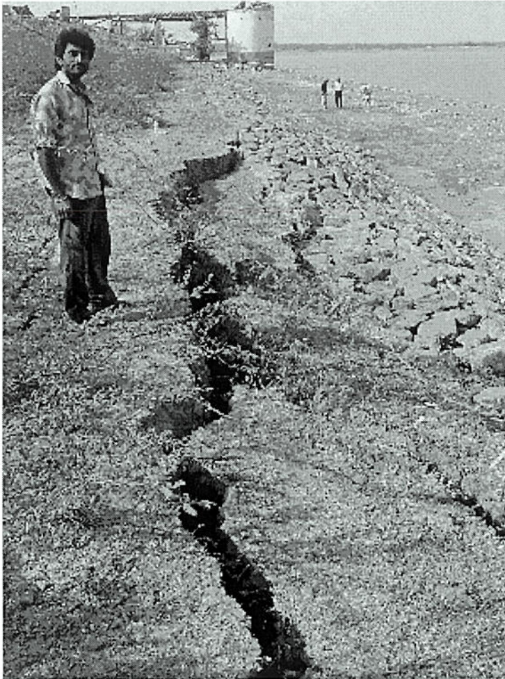
Lateral spreading at the toe and along the lower upstream face.
