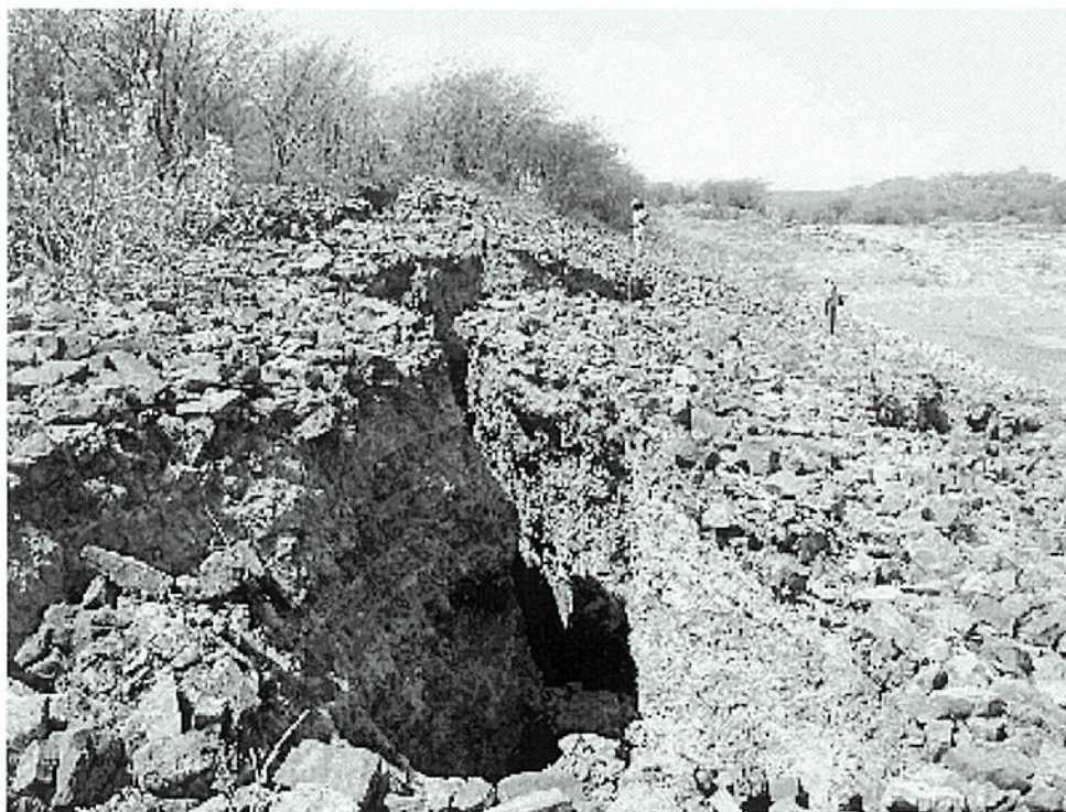
Large cracks on the upstream face.
