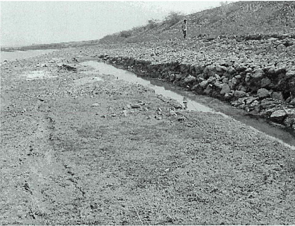
Lateral spreading resulting in a down-dropped section.
