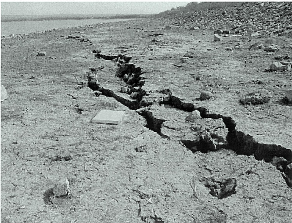
Cracking here associated with liquefaction along the upstream toe.
