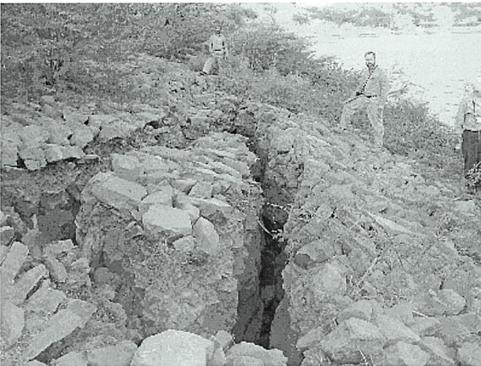
Cracking was observed on the upstream face of the dam up to 2m deep and 0.75m across.
