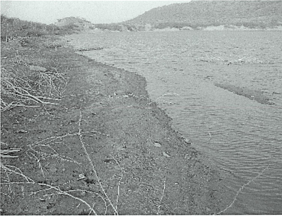
Toe bulging of silt and clay material.
