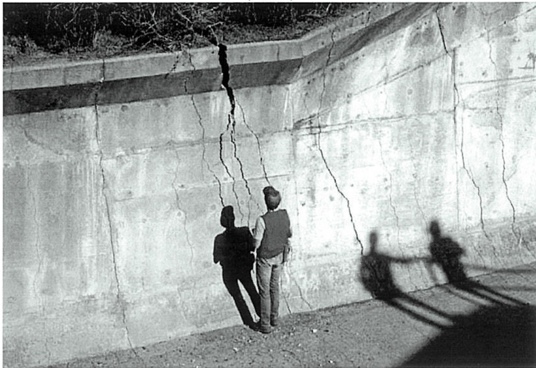
Photo 2 Cracking of Spillway Walls at Austrian Dam (U.S.G.S)
