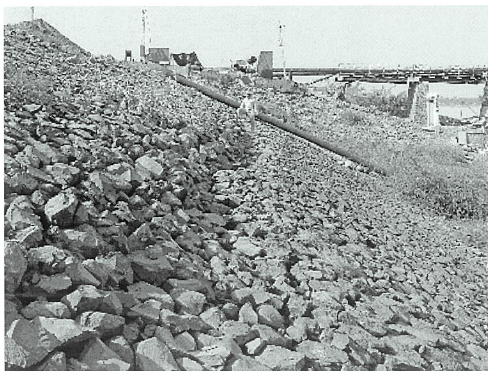
Failures on the upstream face with scarps on the order of 0.75m high.
