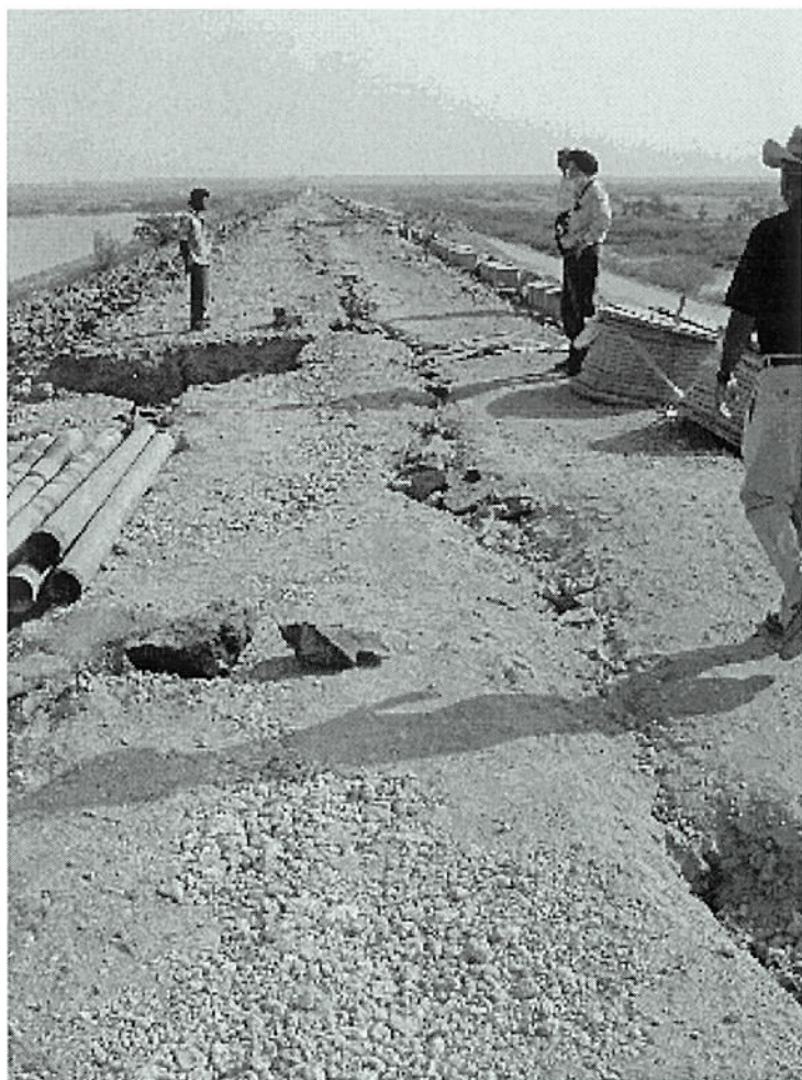
Tapar dam is the most important dam to the region, supplying drinking and agricultural water to the surrounding urban and rural cities and towns. Longitudinal crest cracking up to 1m wide and 300m long was observed.
